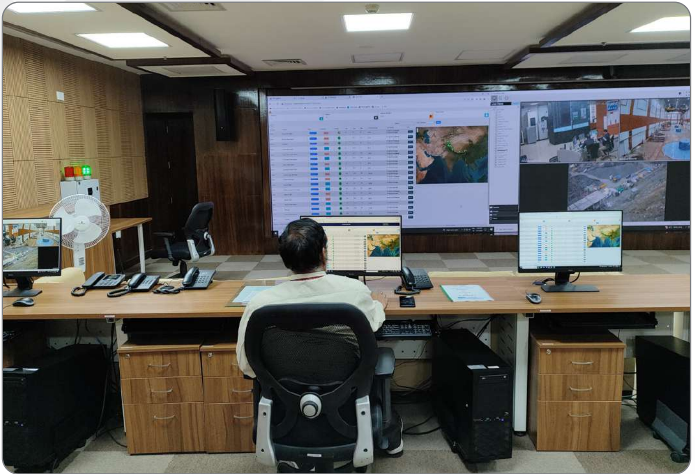
Master control room for EWS at NHPC, Faridabad
