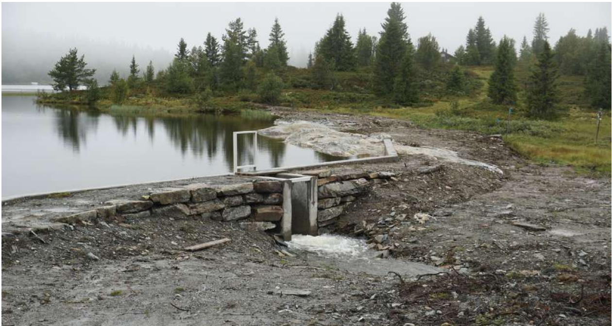
The old stone masonry dam after modifications completed, the measures increased the dam height by 0.5 meter and established a new gate and threshold, with automatic monitoring of the lake level.
